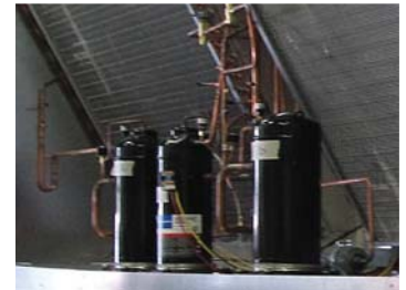
Dehumidification Circuit - Meets Standard 62.1 & 90.1
