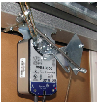
Figure 5. Model CAUA Damper Motor and Linkage Inside Mixing Box
