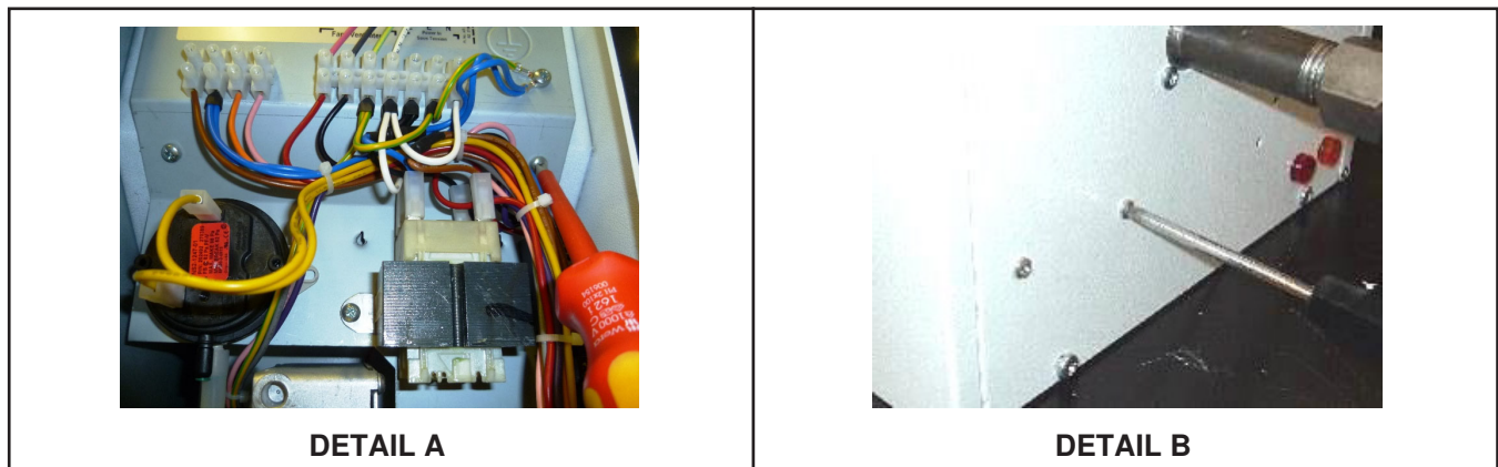
Figure 29. Pressure Switch Removal
